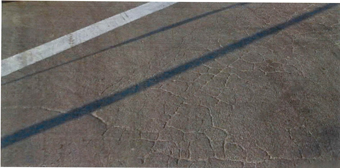
Photo 1. Rutting and cracking along Kuna Mora Road
